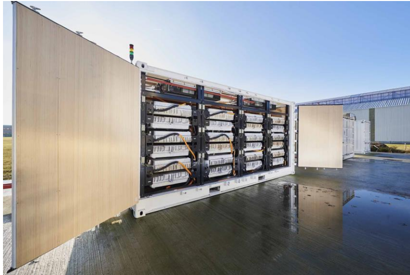
Figure 15. The E-STOR battery ESS by Connected Energy. Reprinted with permission by [81].
