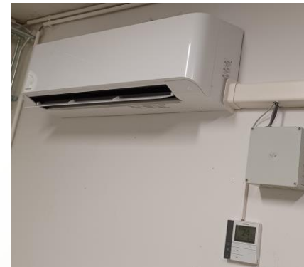
Room temperature and humidity control
